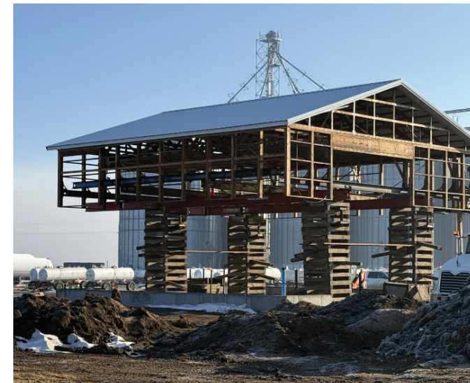
The NH 3 site just west of Belgrade saw some changes with the installation of a new rinse pad area for agronomy equipment.
