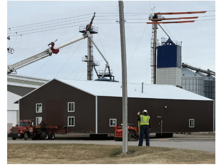
Our mechanic’s shop building was moved to the west side of the main office and is the future home of the Energy Shop.
