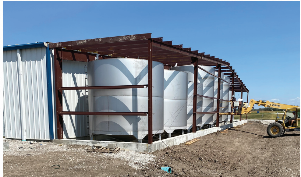
73,000 gallons of chemical storage were added in DeWitt, NE.
