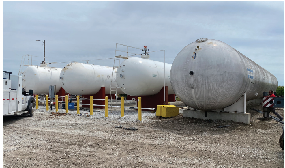
Four new 60,000-gallon NH 3 storage vessels were added throughout our territory.
