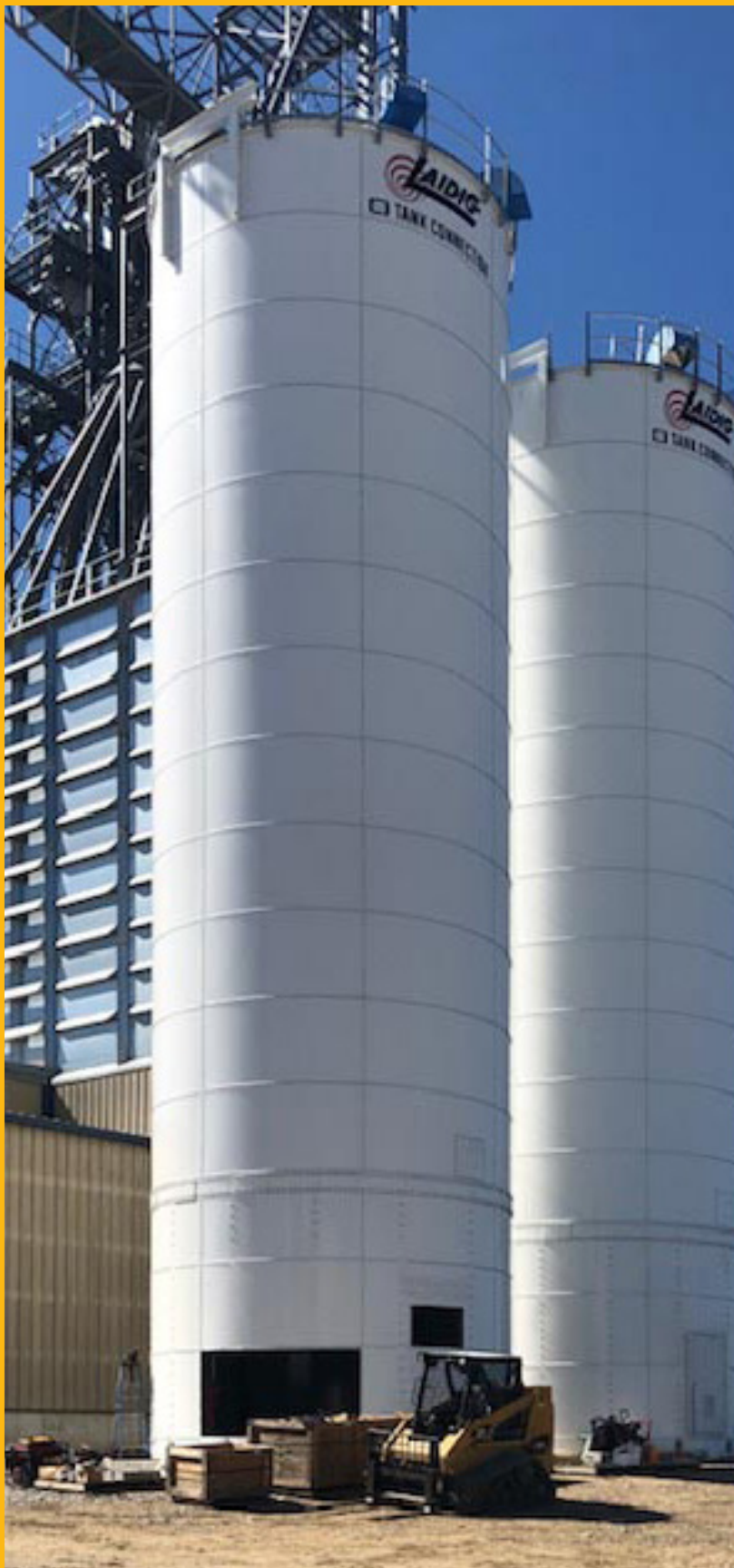
Two new tanks were constructed at the Sunbury, Iowa, feed mill. These additions will provide much-needed storage space for ingredients to keep the mill operating efficiently.
