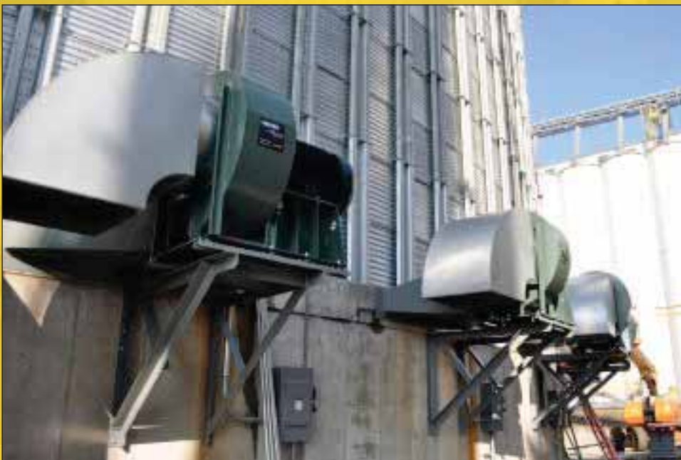
Three of eight Rolfes@Boone 125-hp centrifugal fans equipped with silencers.
