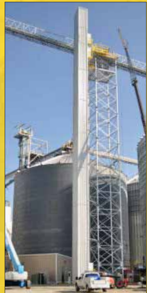
A new Harris Companies manlift being installed to run from ground level up to a Hawthorne-Seving catwalk.
